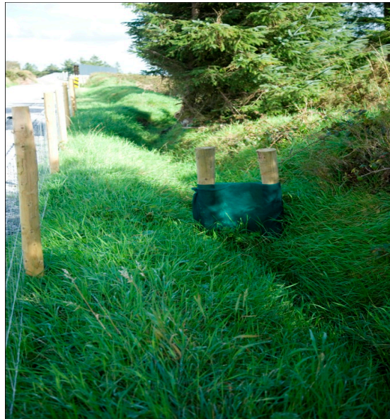
Figure 3-5: Silt trap across grassed swale
